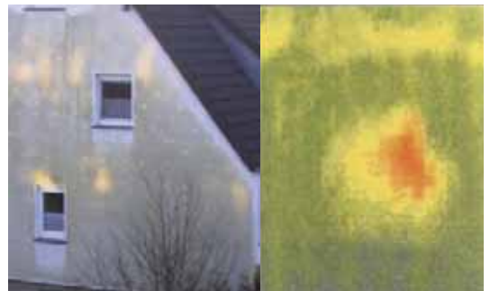
Thermal bridges caused by fixings commonly used to fix EPS.
